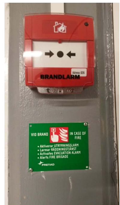
Hallway fire alarm
